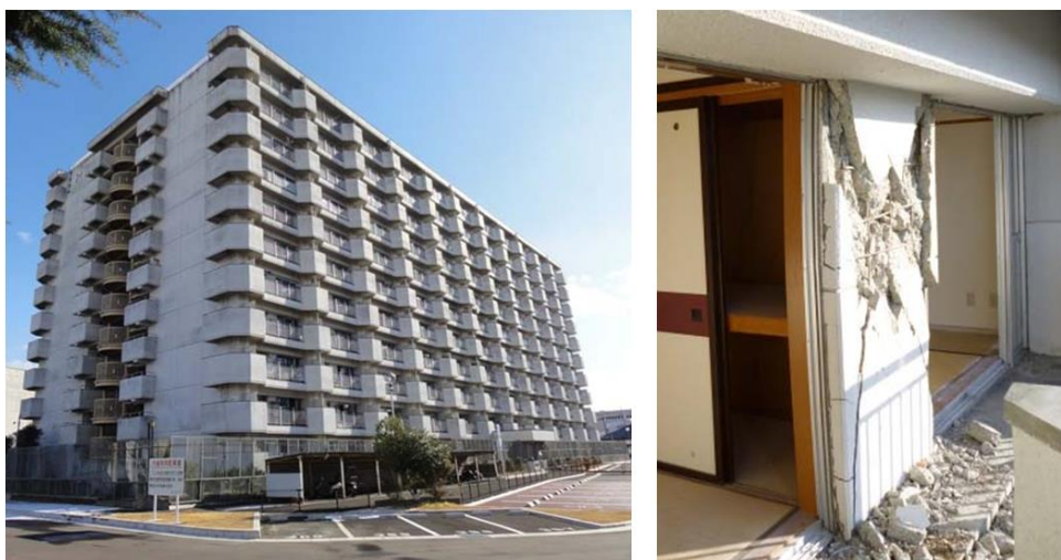
Fig. 3 – A 12-story steel reinforced concrete apartment in Sendai after 2011 Tohoku earthquake and was later demolished (Courtesy of Professor Y. Sanada at Osaka University)
