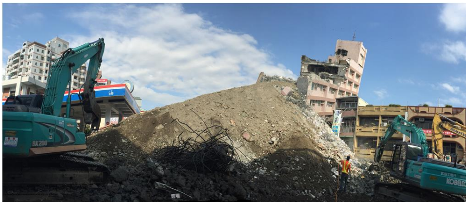
Fig. 2 – Temporarily piled slope for excavators to demolish a collapsed frame building in Tainan earthquake
